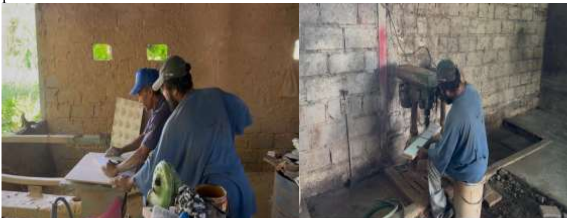
Figure 2. The Craftsman Didn't Use Personal Protective Equipment (PPE)
